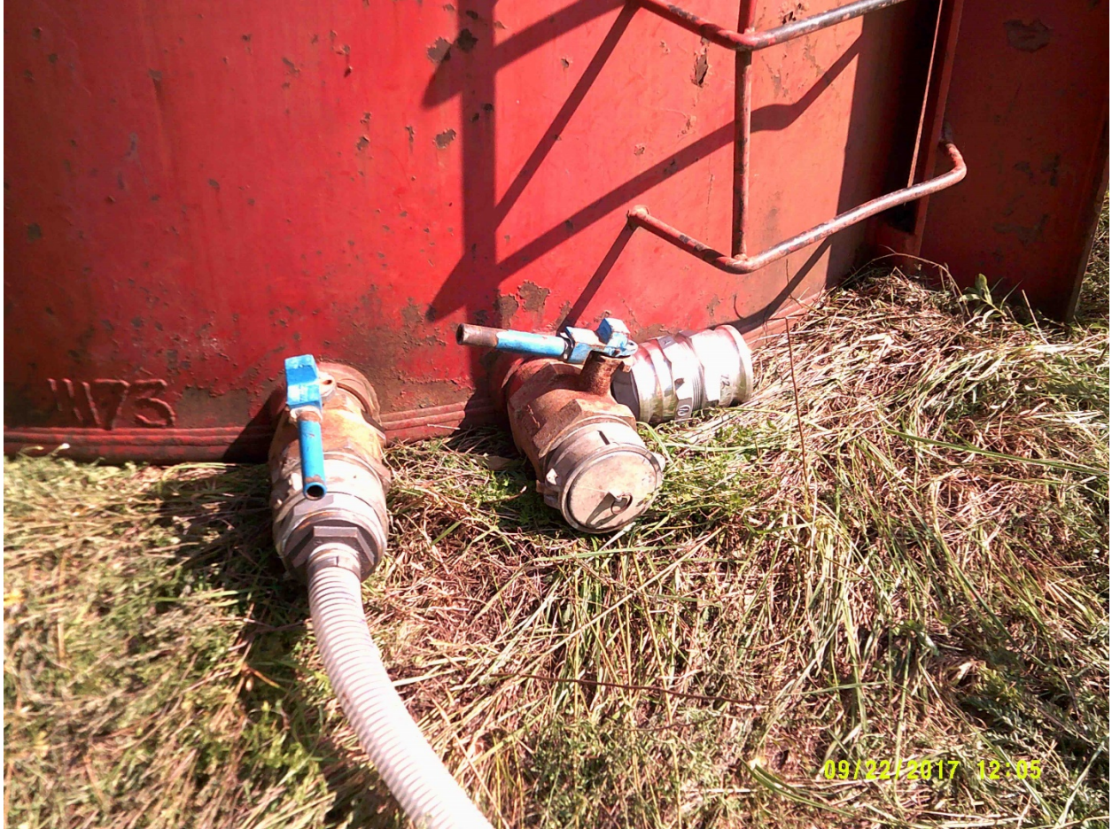
Figure A-8: Intake Hose and Water Tank
