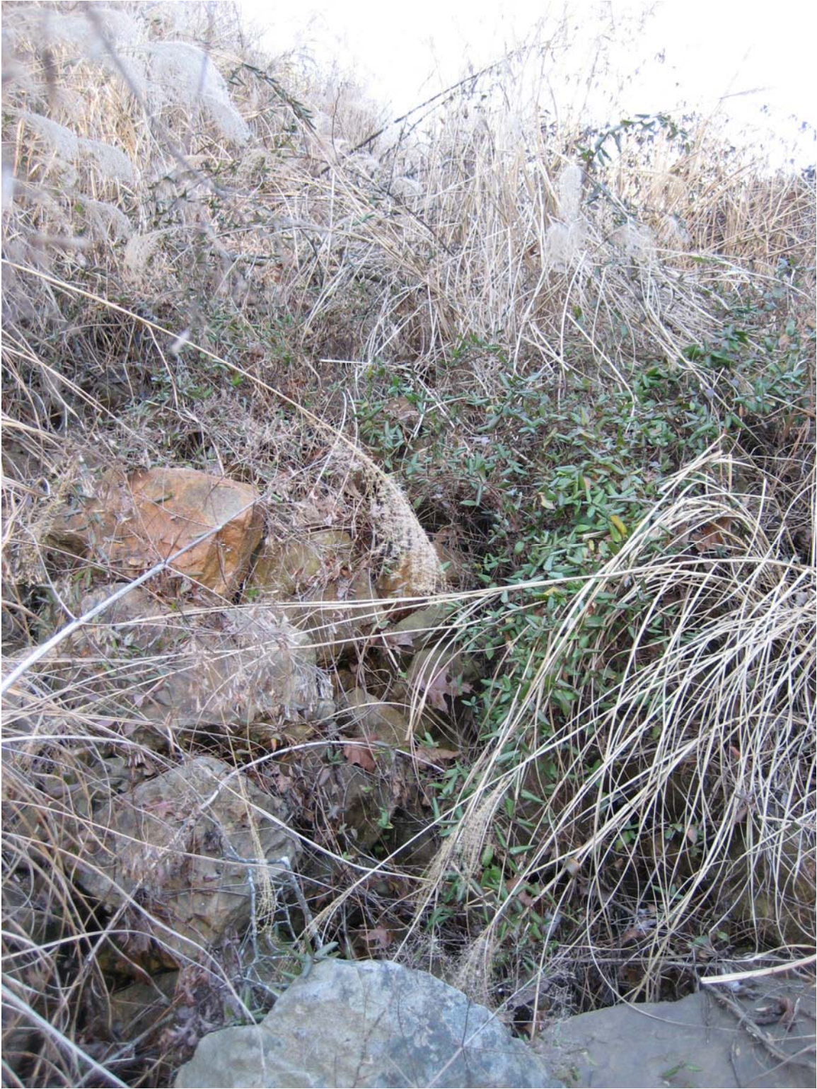
Figure 6: Boulders Down-Gradient of Principal Spillway.
