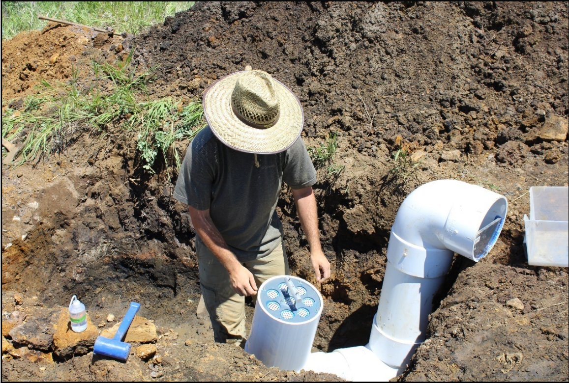
Figure 4.5: Second cartridge installation to the modular treatment system.
