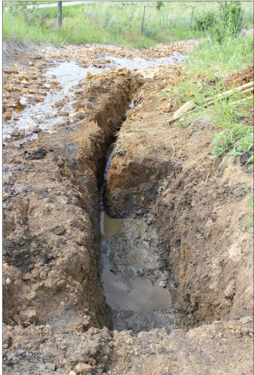
Figure 4.2: Hole and drain excavated for the modular treatment system next to ARD channel.
