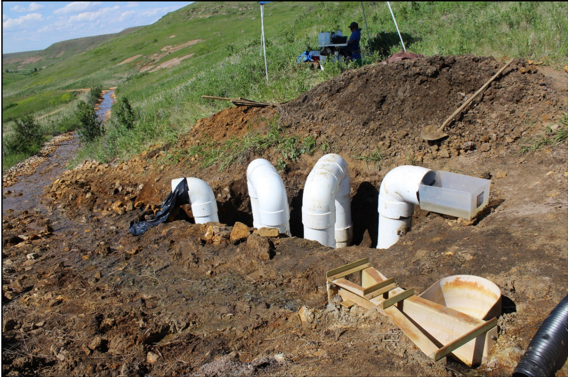
Figure 4.10: Entry-weir connected to the modular treatment system.
