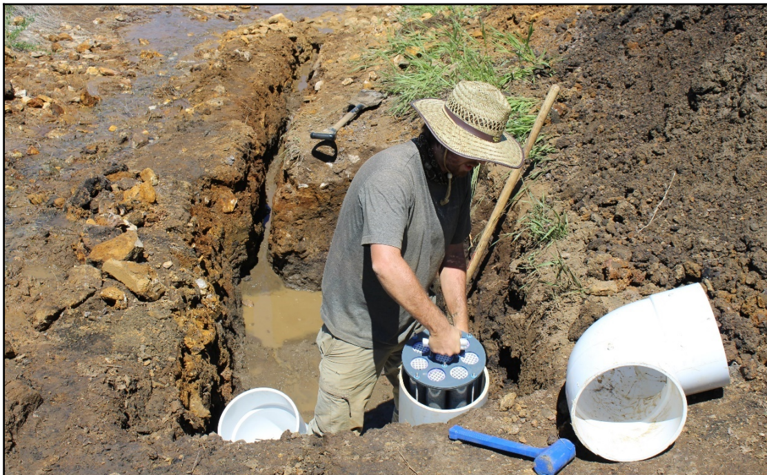
Figure 4.4: First cartridge installation to the modular treatment system.
