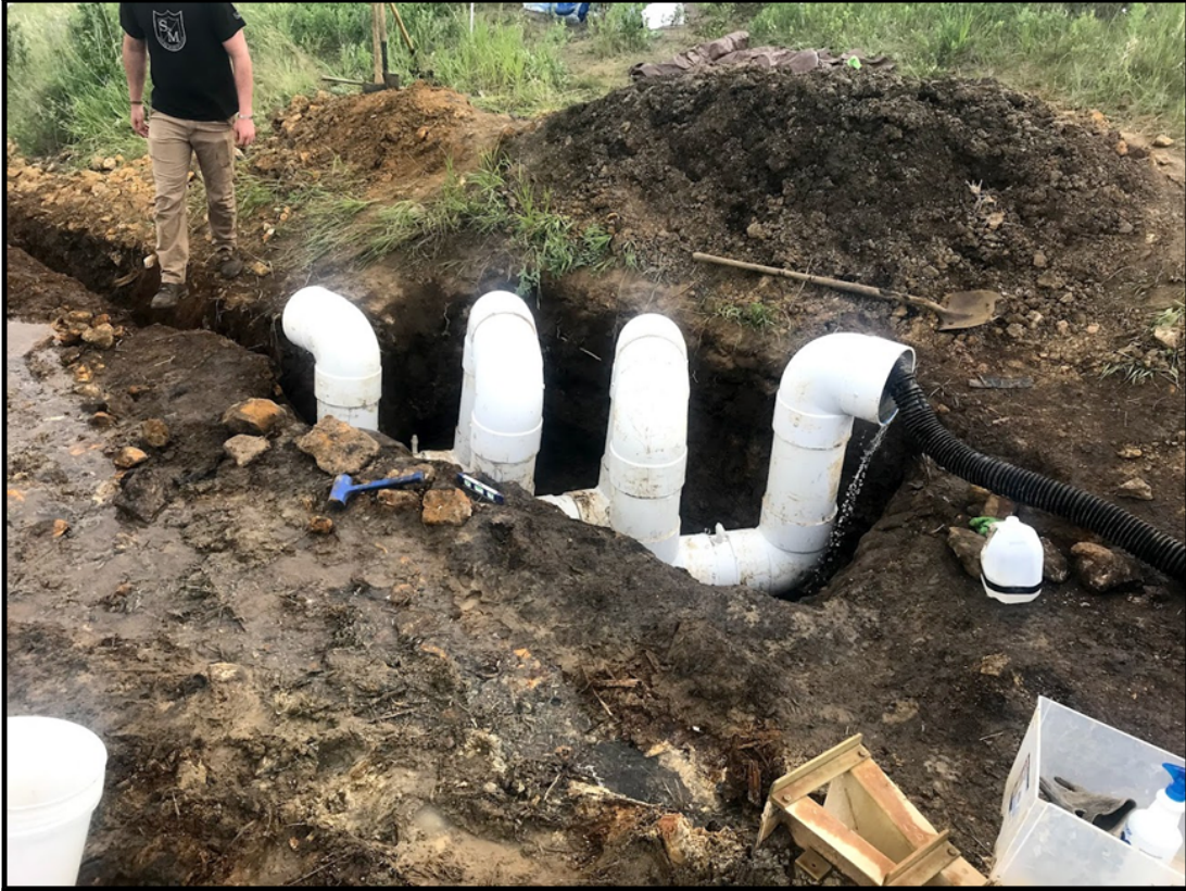
Figure 4.11: Entry-weir replaced with gutter drain due to leakage.
