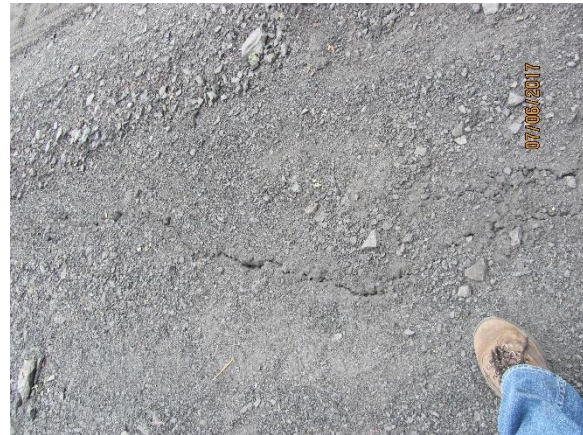
(b) Cracks formed due to blasting
