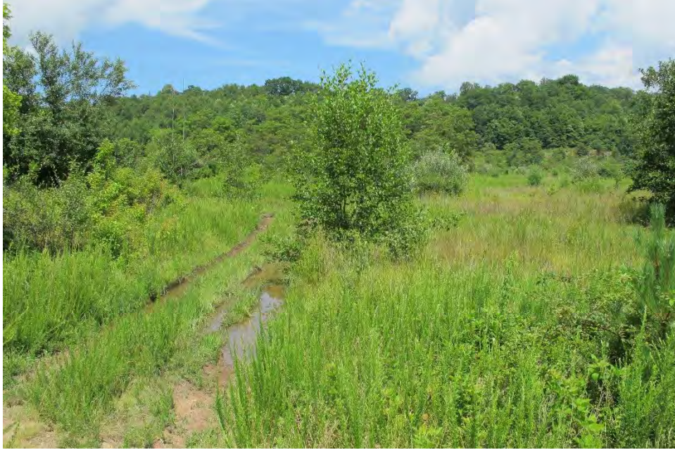
Figure 34. R070700 Differential settlement of impoundment cap.
