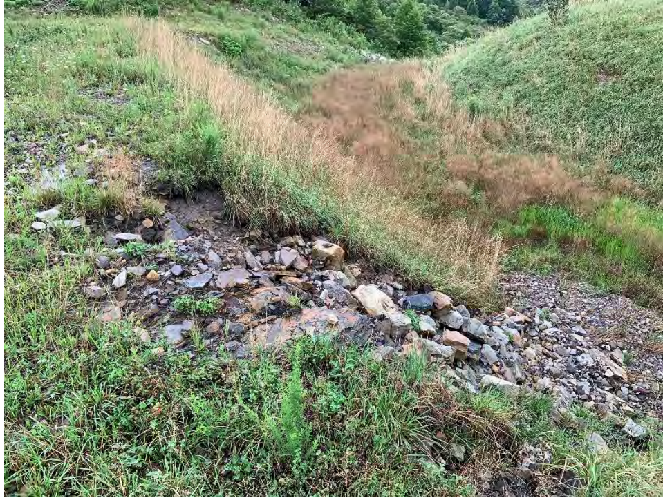
Figure 47. S024076 Eroded hillside adjoining open channel ditch.
