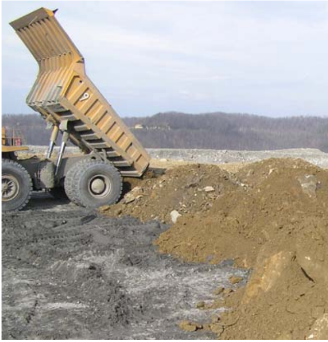
Photo 1. Loose dumping a topsoil substitute over a compacted subsurface on a West Virginia surface mine. The topsoil substitute material is being dumped in closely spaced piles and will be graded using only a single dozer pass. The final surface will be revegetated with a tree-compatible groundcover and trees will be planted in the loose topsoil substitute materials.
