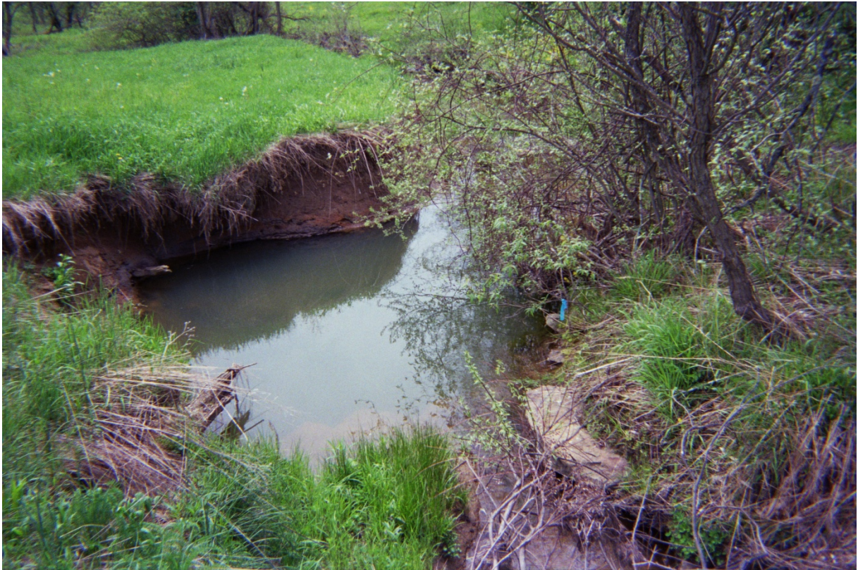
Figure 44. Stream F, PA. Pothole located between 1080 (329.2 m) and 1090 feet (332.3 m) downstream, over the upstream quarter-panel of longwall panel 1. This ‘pot-hole’ has formed at the base of the higher gradient cascade reach observed entering the pot-hole at lower right corner of the photo. Stream erosion has widened and deepened the channel at this location due to effects from longwall subsidence.
