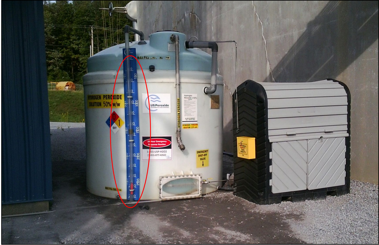
Figure 7. Photo of POLY double-walled hydrogen peroxide tank with level indicator in red circle.
