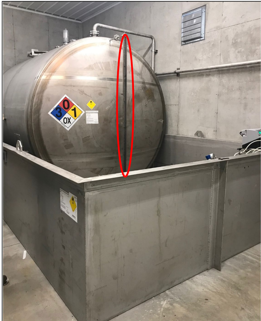
Figure 3. Stainless Steel Storage Tank for Hydrogen Peroxide with steel secondary containment. Note the ventilation fan in the upper portion of the photo. In the event of a leak ventilation fans will greatly assist in removing peroxide vapors from the building atmosphere.
