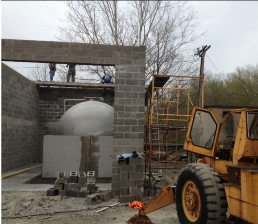
Figure 4. Photo of the construction of a concrete block storage building with stainless steel tank located in the building.
