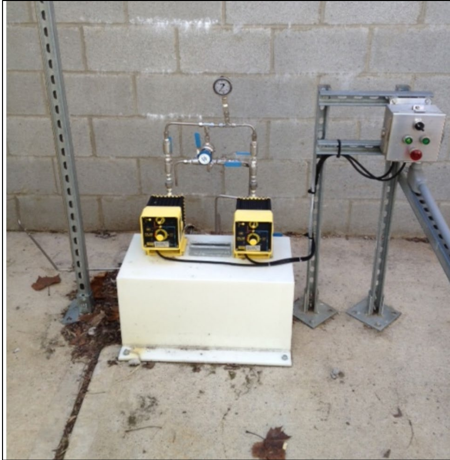
Figure 11. Photo of a two-pump hydrogen peroxide dosing skid and associated stainless-steel tubing. Note the presence of organic matter (leaves) in the vicinity of the diaphragm pumps. This is a situation should be avoided and immediate correct action is needed as a leak of peroxide will result in combustion of any exposed organic material.
