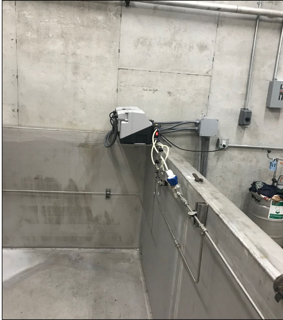
Figure 8. Picture of stainless-steel and polyethylene tubing associated with Dosing Skid. Note pumps and piping are mounted inside the secondary containment structure.
