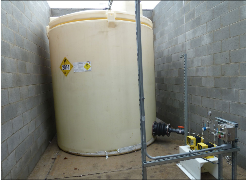
Figure 6. Double-walled POLY Tank and associated two-pump Dosing Skid. Storage Tank is placed on exterior concrete pad within concrete block structure.
