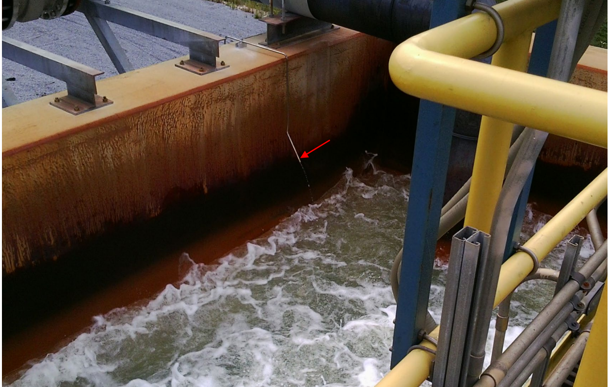
Figure 12. Photo of the hydrogen peroxide dispensing (red arrow) into the mine drainage water. 90 gallons per day of 50% peroxide is being utilized to treat this 4500 gallon per minute abandoned underground mine discharge.
